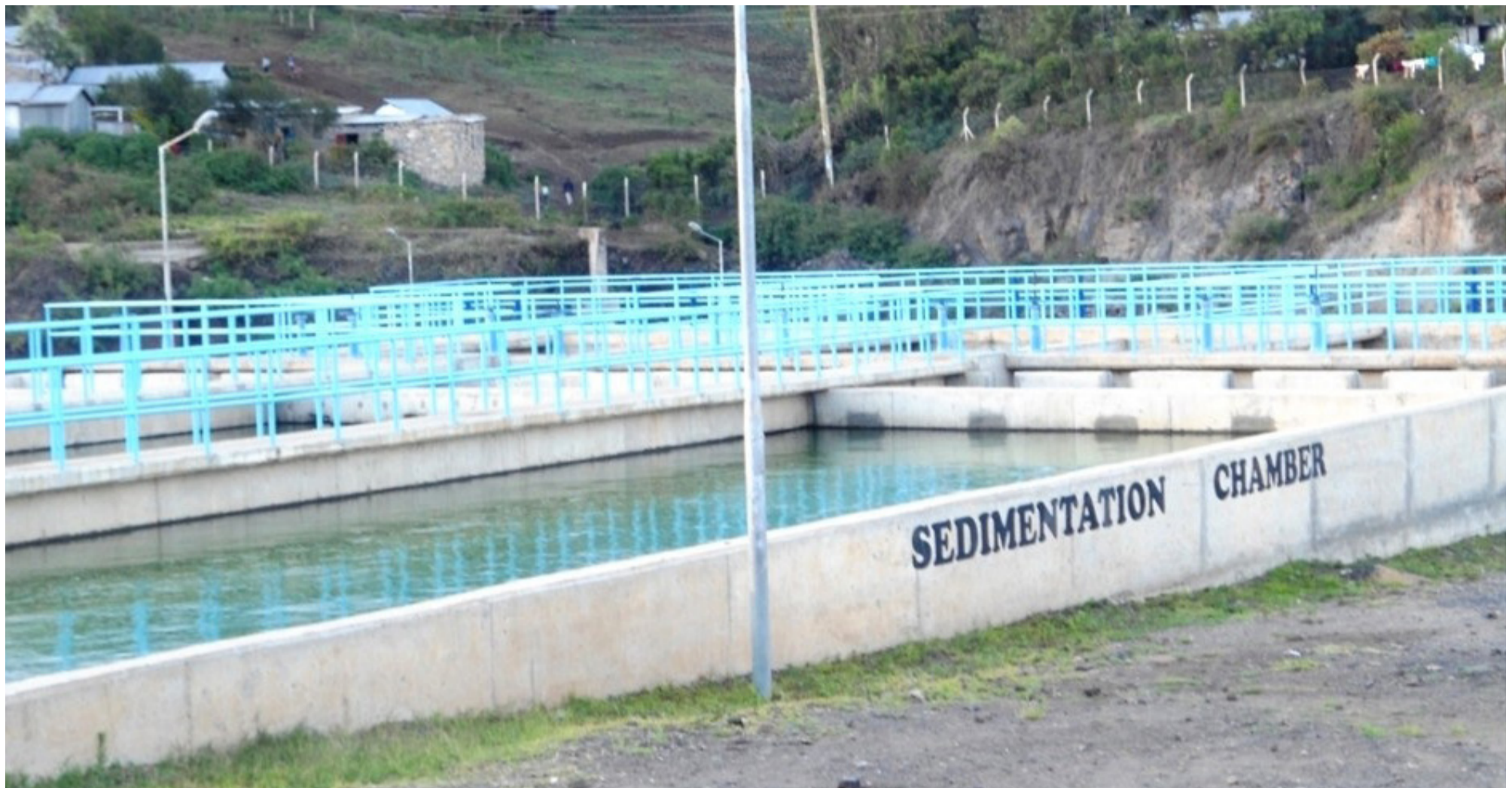
Sedimentation Chamber at the Kiserian dam which is located along the Kiserian River about 2kms from Kiserian Township and supplies water to Kiserian, Ongata Rongai and parts of Ngong' townships. PHOTO | NWH&SA.
