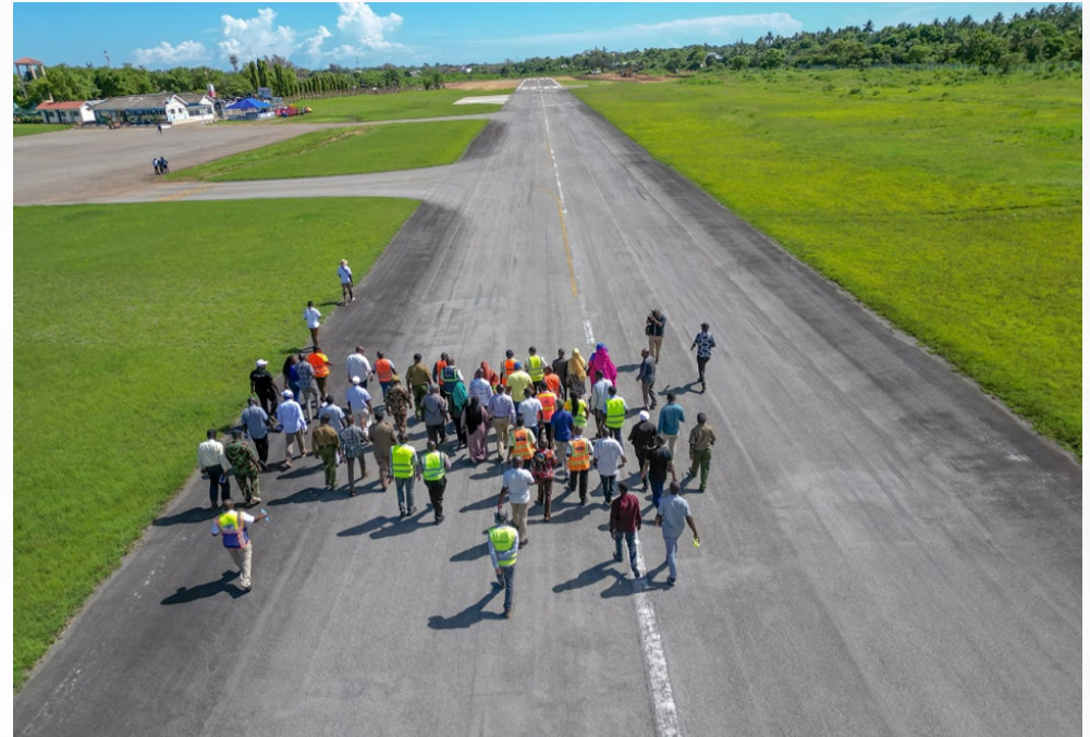
The then Roads and Transport Cabinet Secretary (CS) Kipchumba Murkomen during a visit to the Diani Airport (formerly Ukunda Airstrip) to inspect and assess the progress of the construction of the concrete Turn pad, runway and runway strip on November 14, 2023. PHOTO | Onesimus Kipchumba Murkomen/CS/FB
