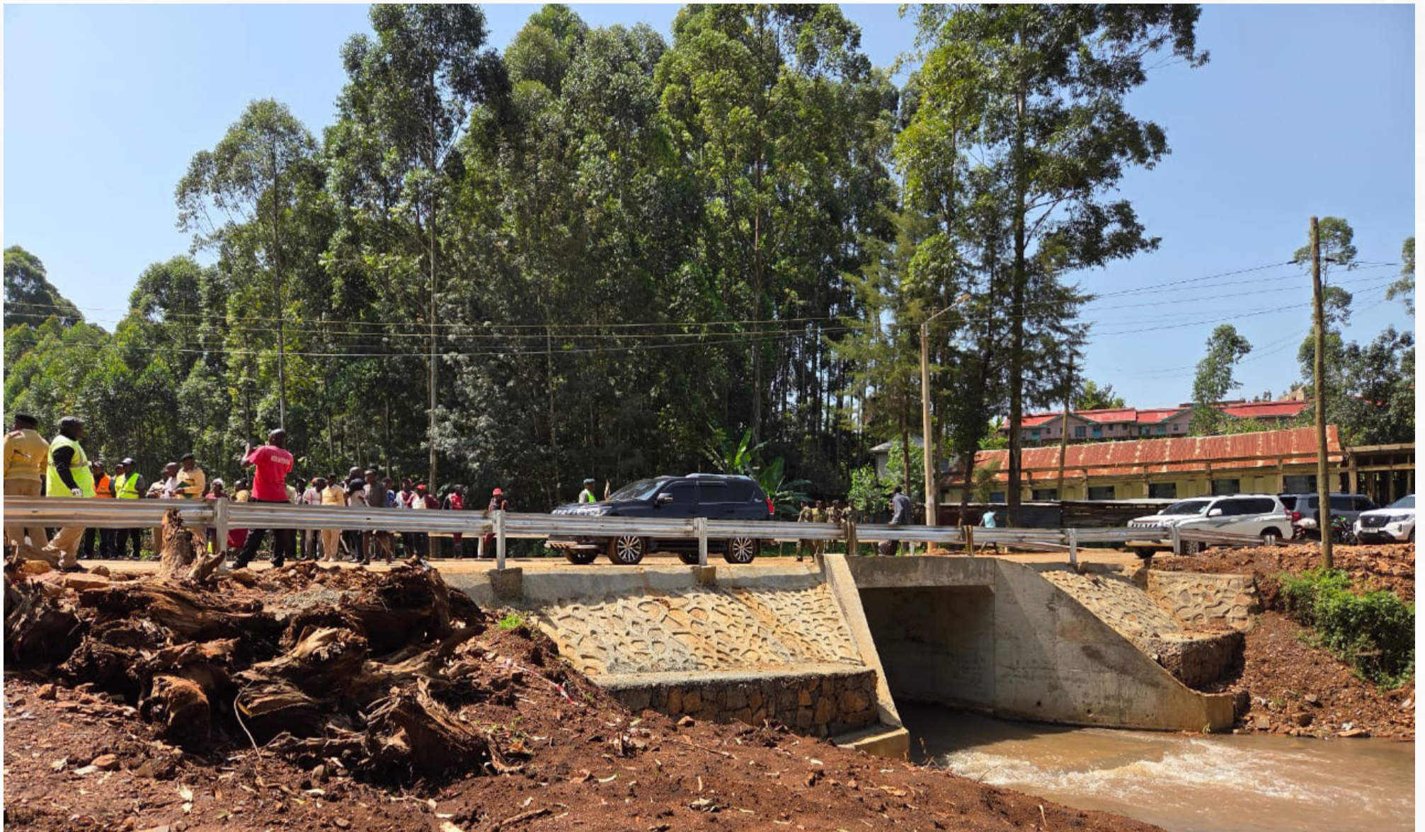
The Nyamache Bridge - part of the Nyacheki-Riokibeni-Nyamache Box Culvert on Road C957 project in Kisii County on June 24, 2025. PHOTO | GDU
