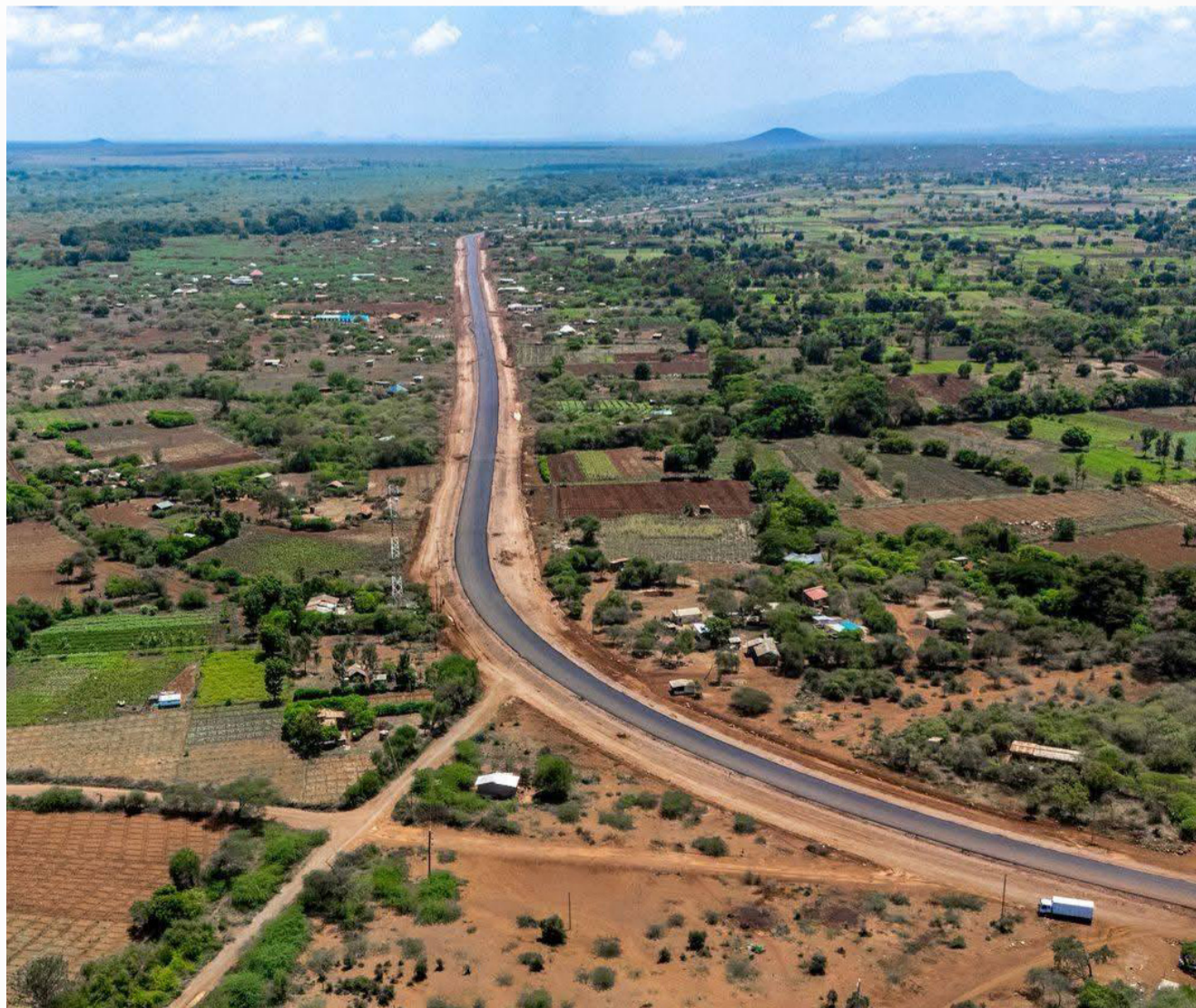
An aerial view of a section of the 33-kilometre-Ksh4.1 billion Mteza-Kibundani road on February 19, 2026. PHOTO | Office of the Deputy President
