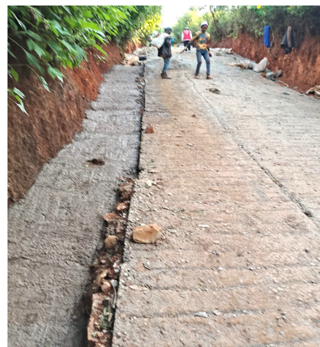
A Section of the Gatumbi-Githima road in Gachochi location, Kinyona ward in Kigumo on January 7, 2025. PHOTO | Irungu Kang'ata.
